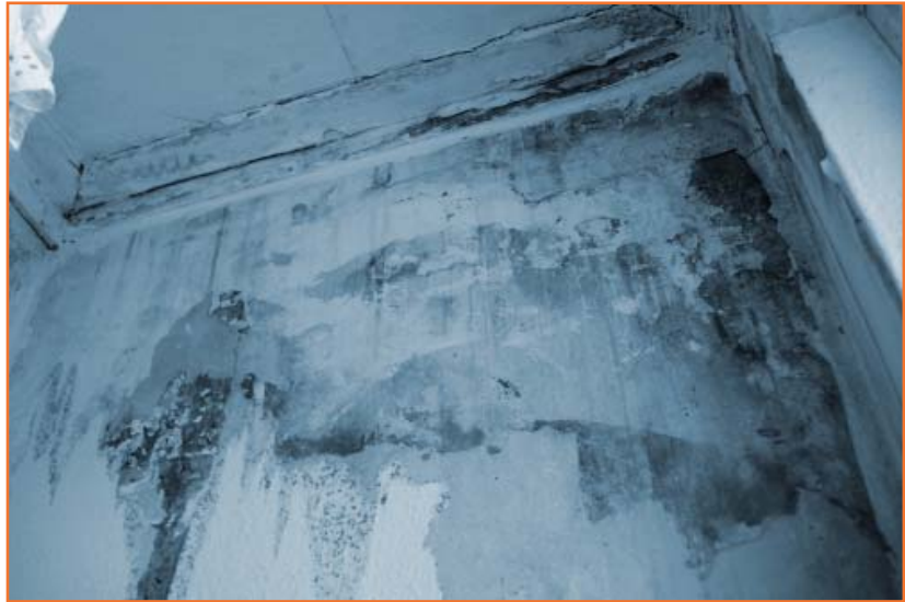
Extensive damp/mould problem on an internal wall
