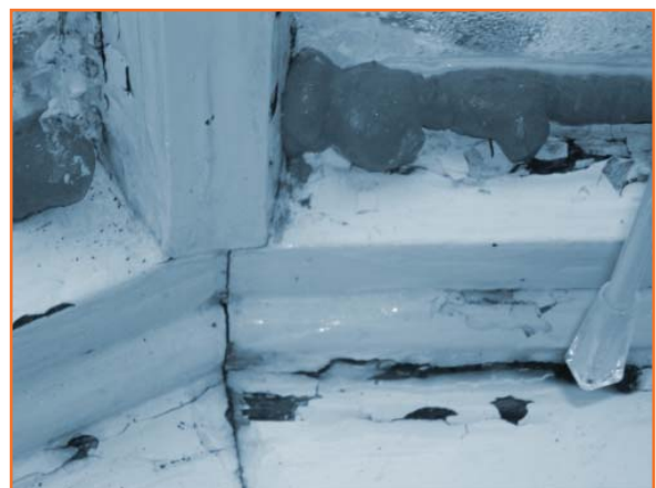
A window repair issue
