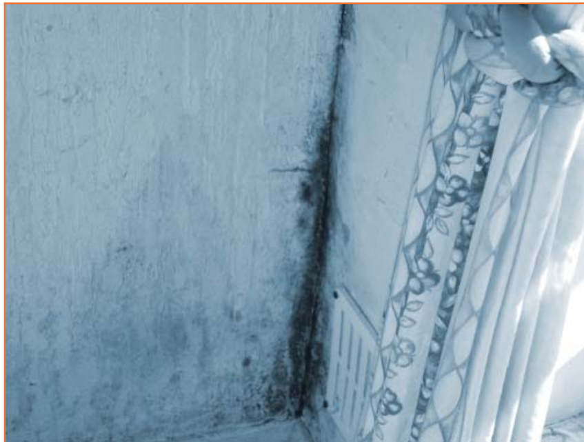
Damp/mould problem found during an inspection
