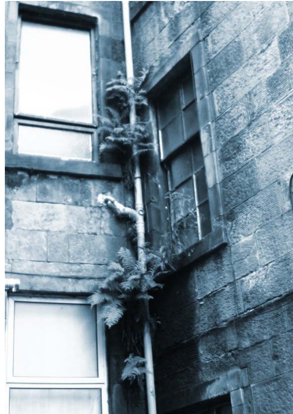
Example of a common parts repair issue
