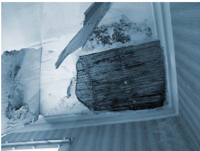
Ceiling complaint in a tenement property
